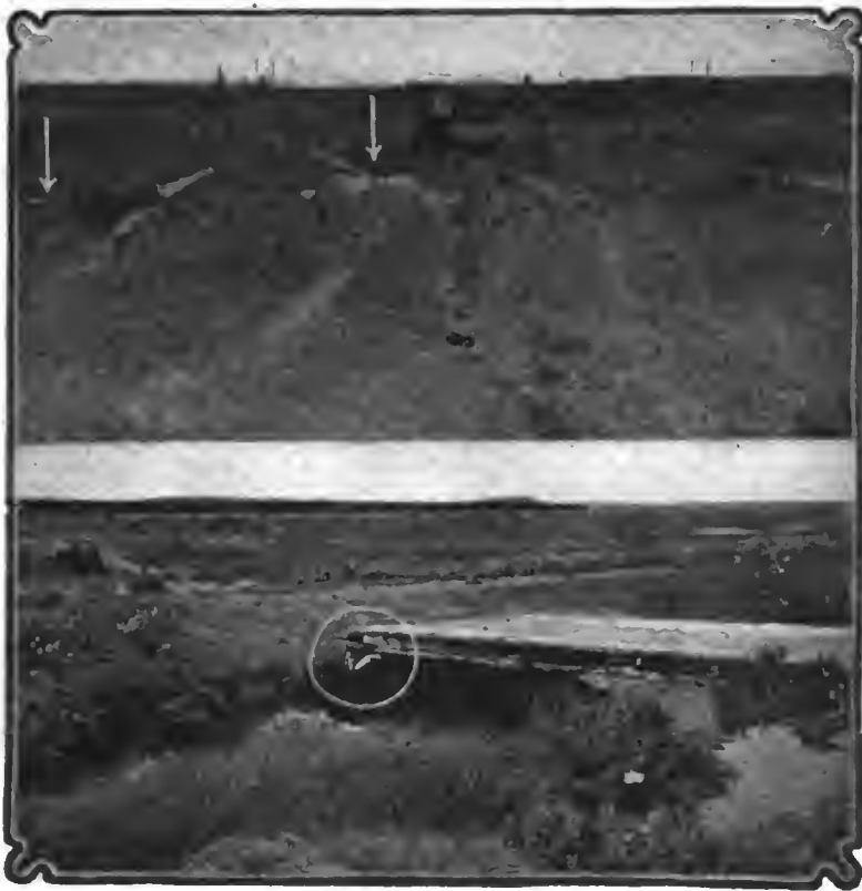
Upper—Two cloudbursts had changed this alkali road 4 miles east of Laramie into a swamp hole for a distance of 8,100 feet. Three distinct sets of wheel tracks may be seen where automobiles have tried to avoid the pitfalls of those who had gone before. This one bad spot in a distance of many miles could be eliminated by using the earth on the sides to build up the center, with a cross-culvert to take care of the water that runs back and forth on the low ground at each side. It took a car 1 hour with outside assistance to make this 100 feet. Vertical arrows indicate a board over a cross-under drain which was badly choked.
